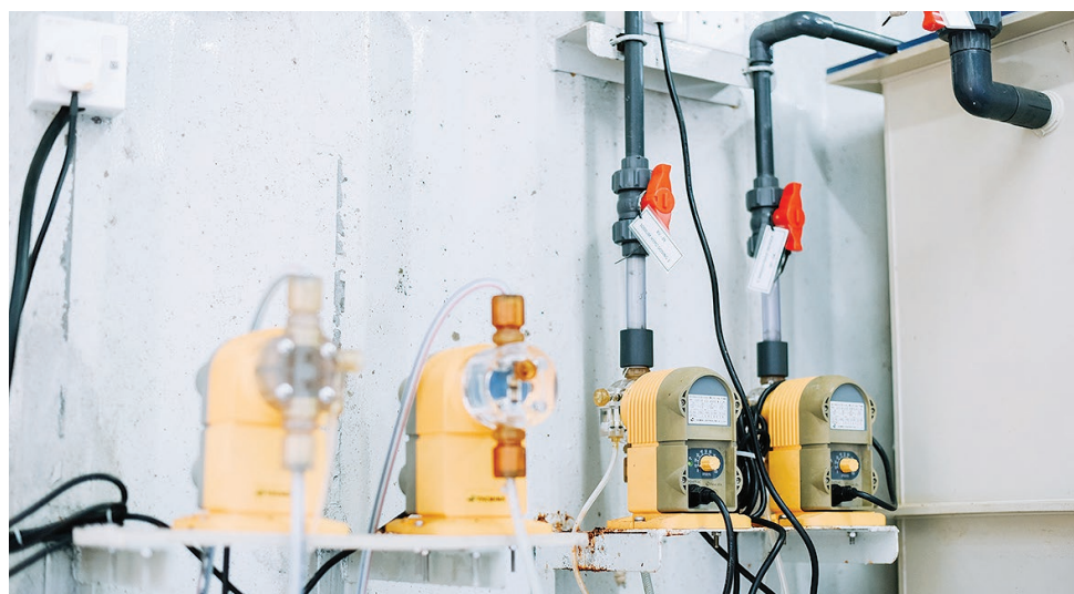
Creativity and innovation have allowed AIR Bhd to use limited space in an unlimited way, such as taking in seawater into SWRO systems from one end and taking out potable water from the other
